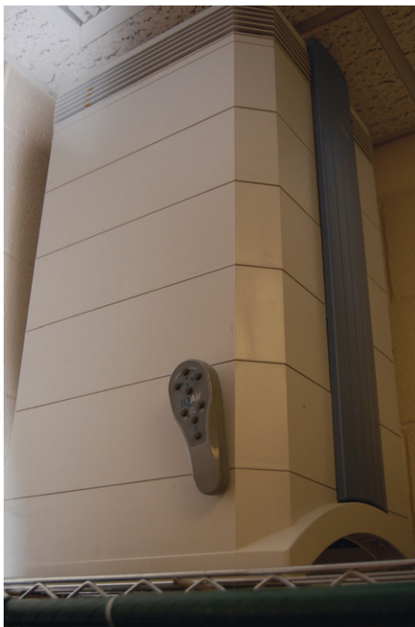
Fig 6.5 An air filtration unit within the avian hospital ward.
